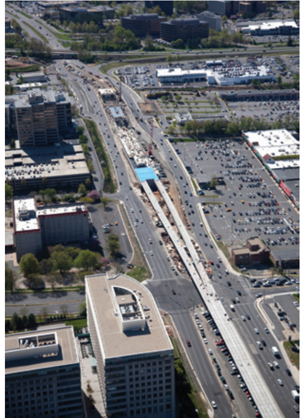
The Silver Line under construction in the median of a highway in Tysons Corner. Photo courtesy of VDOT.
